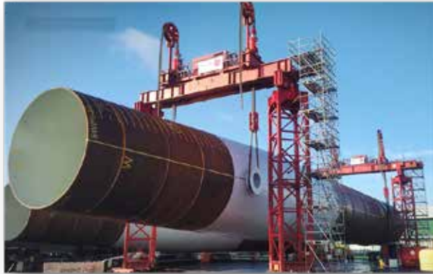
Heavy lifting equipment
